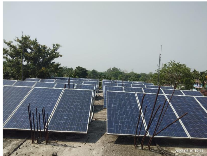
Figure 6: 10 kWp Grid Connected Solar Power Plant
